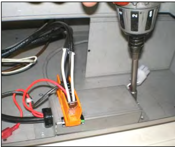
Lamp Transformer housing may need to be moved toward valve.
