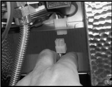
Figure 24: Disconnecting 24VDC to gas valve assy.
