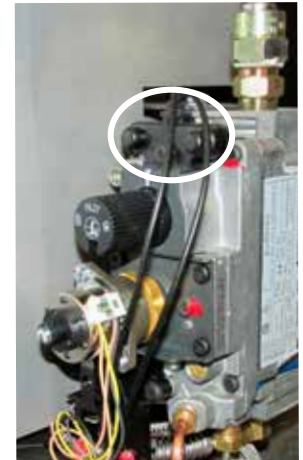
DC Sparker Wires
