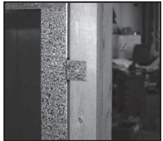
Figure 20: Framing tabs bent out.
