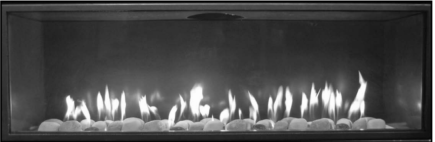
Figure 85: Example of desirable flame pattern.
